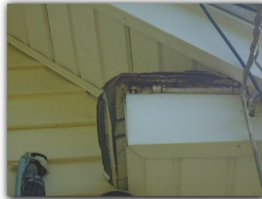
Observed decayed decking.
