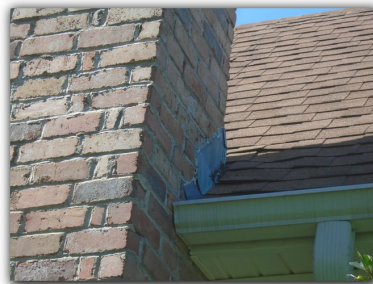
Flashing needs resealing
